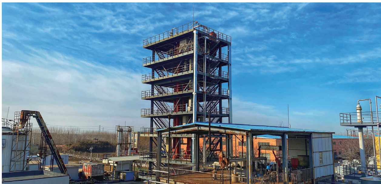
A 1,000-ton scale biomass chemical looping gasification pilot platform that produces green methanol.
